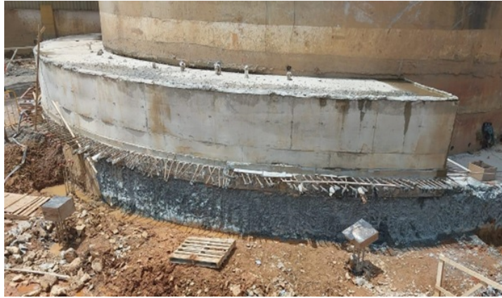
Figure 9 - Construction of the counterweight on the outer face opposite the settlement area.
