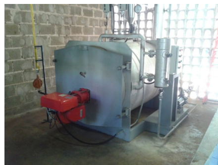
Figure 9 – Boiler used for steam generation in the UR.
