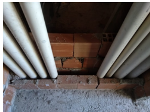
Figure 10 – Shaft for bathroom vertical piping and plumbings.
